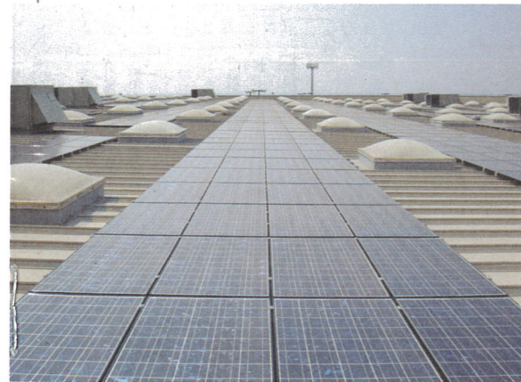
Photovoltaic solar panels and skylights at the Kona, Hawaii location.
